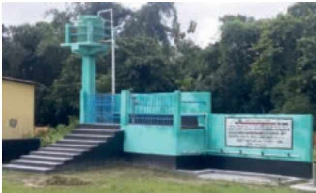
Drinking water facility in school
